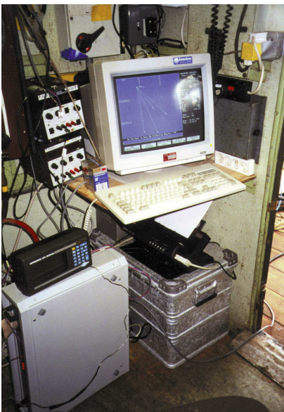
Figure 26: Prototype seismic positioning system used in 1996. (Author)
